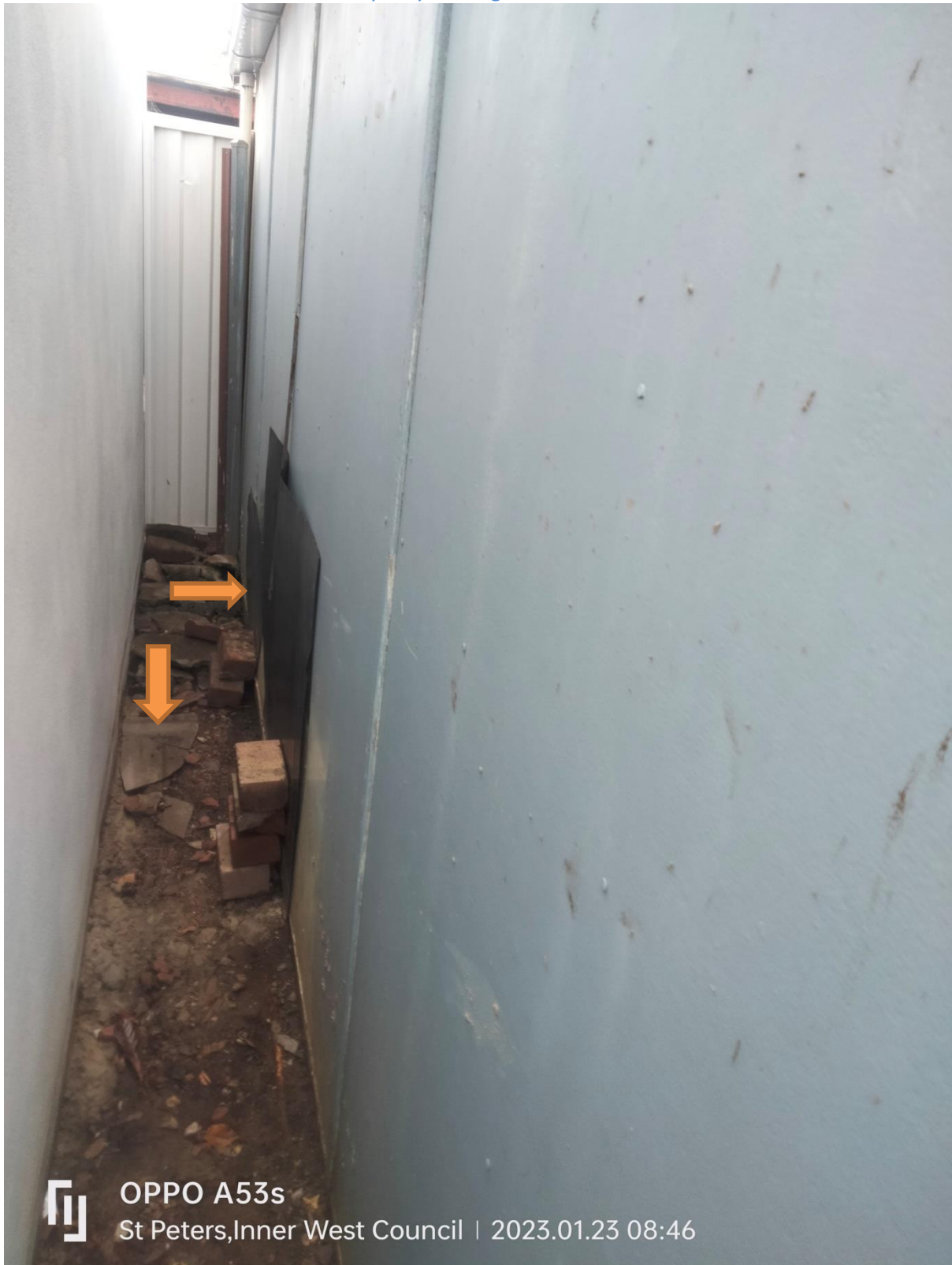
Figure 8 existing impact damage to number 120 garage location, I note asbestos was evident on the floor dividing the two garages.
