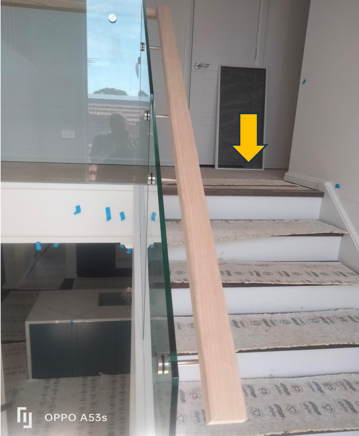
Figure 17 the top of the stairs was noted as squeaking. This is a defect.
