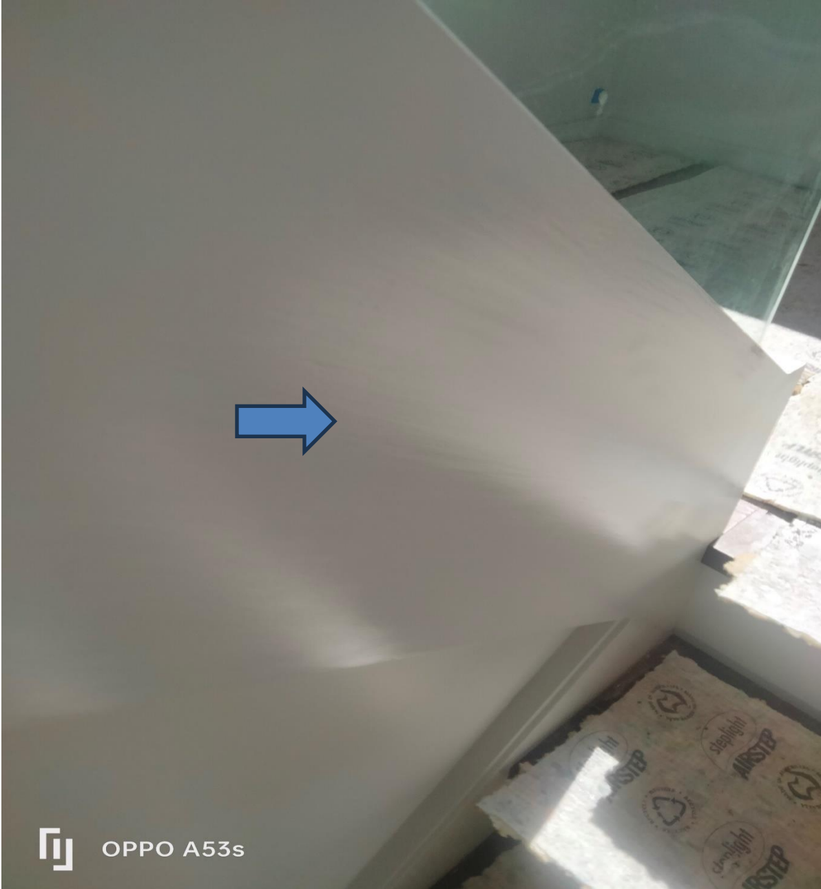
Figure 16 the timber stringer was observed in natural light requiring final coats. Incomplete painting.
