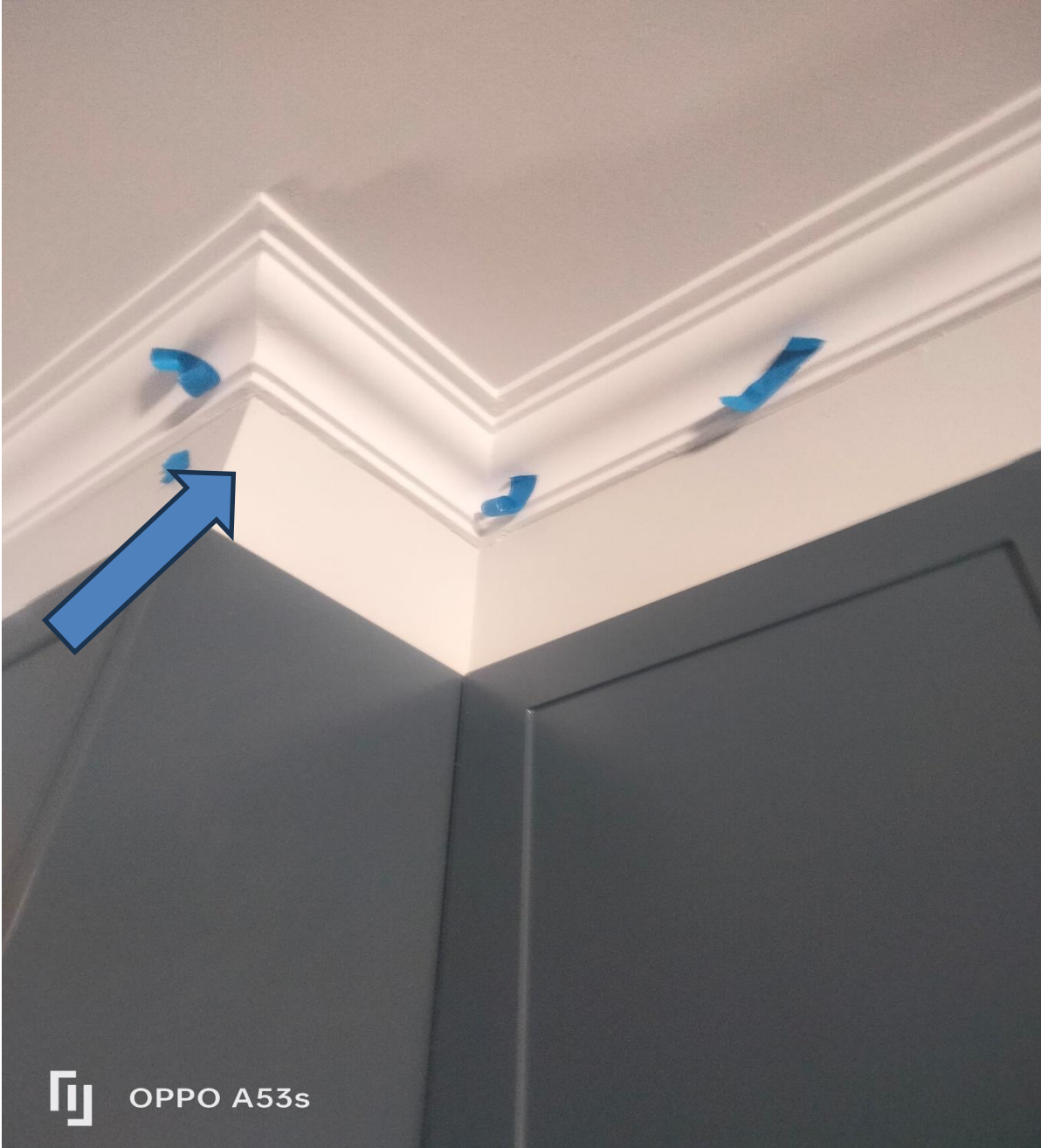
Figure 5 incomplete painting observed throughout the house clearly visible from 1.5 meters away. Incomplete work.
