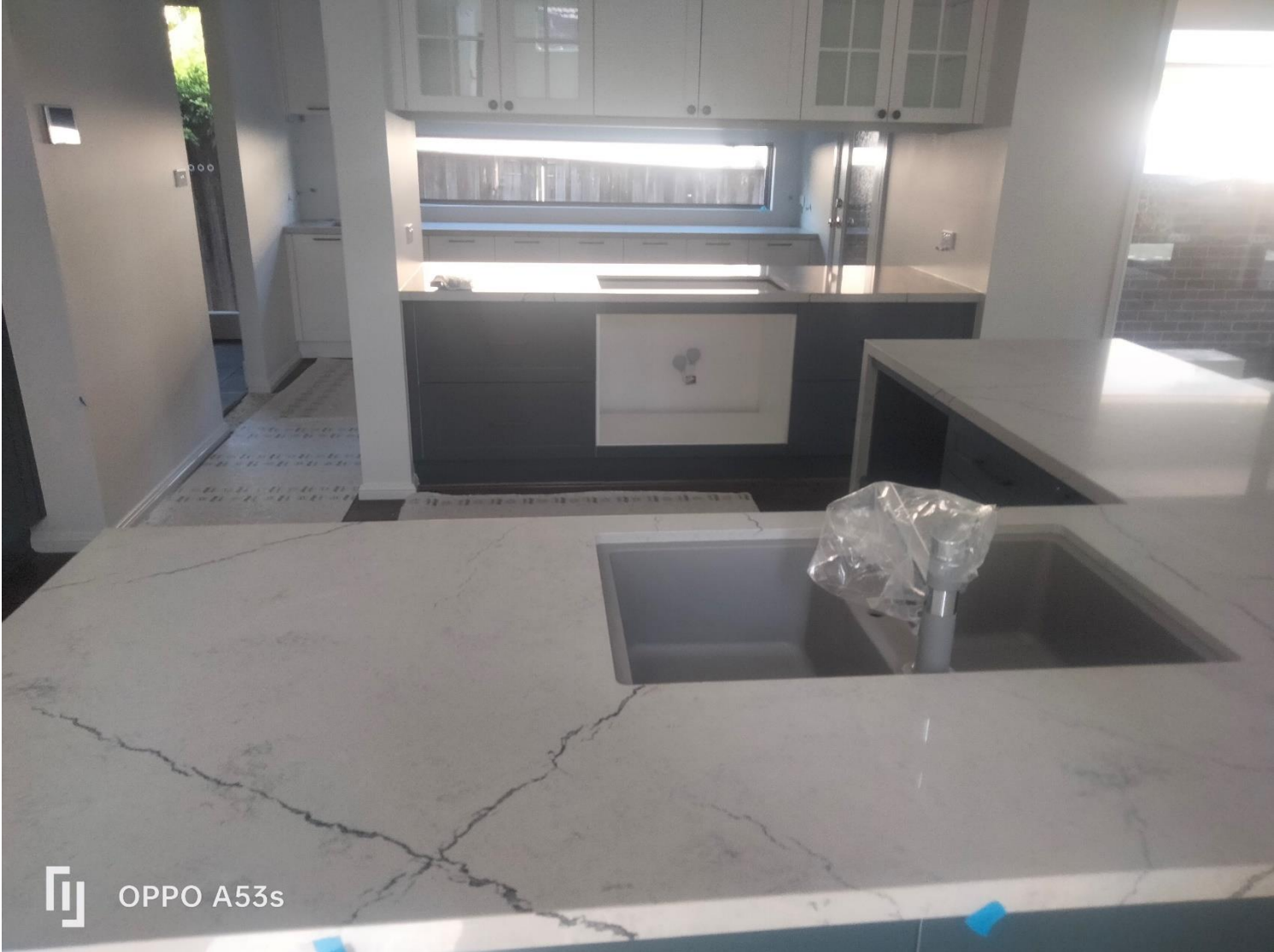
Figure 6 the kitchen benchtop was observed as having blue tape indicating incomplete locations.
