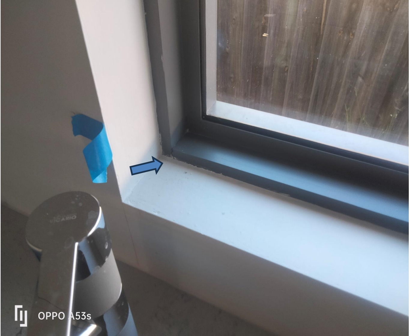
Figure 8 poor kitchen painting to metal frame windows.
