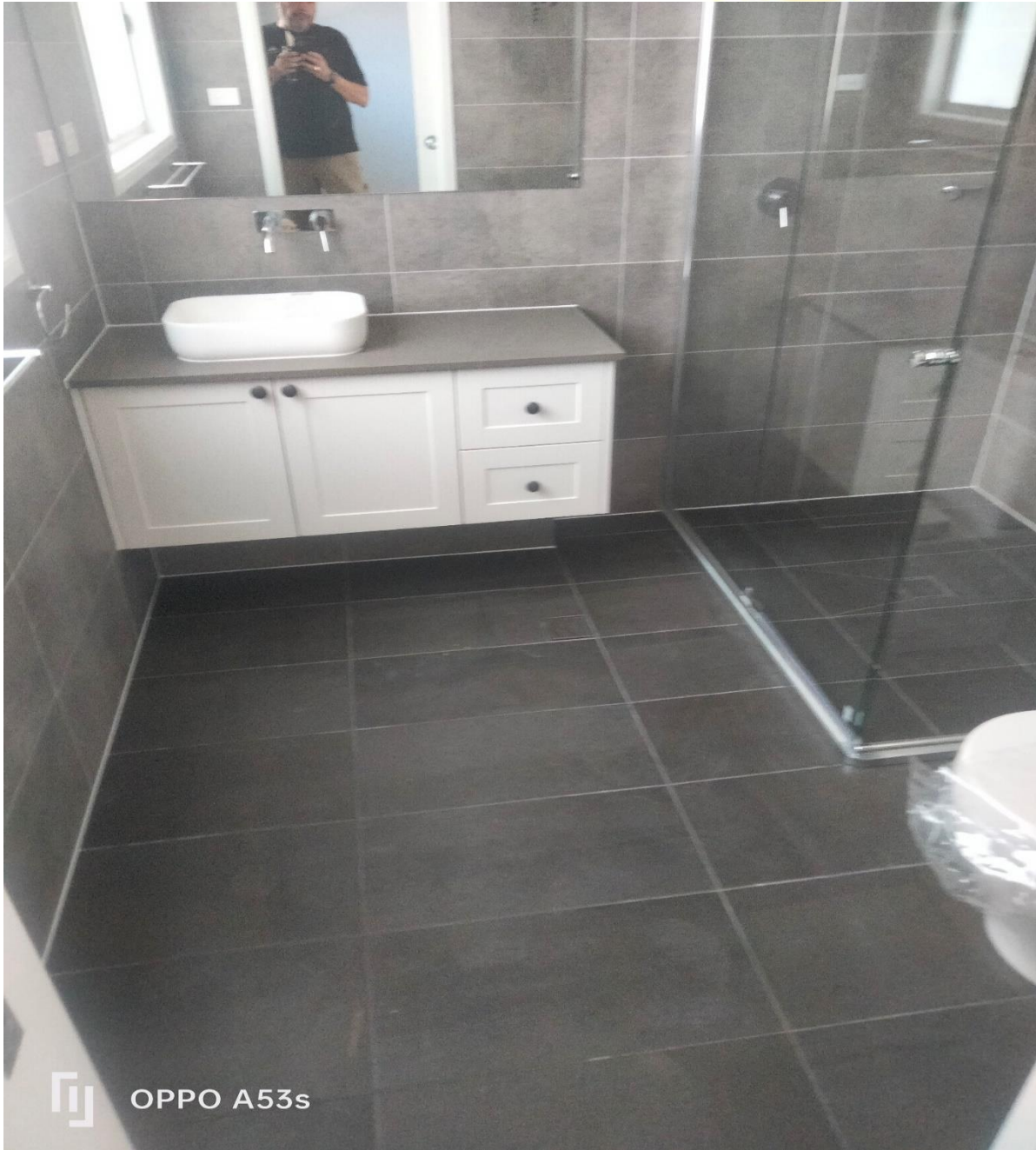
Figure 19 bathrooms were inspected and revealed incomplete works throughout including missing kitchen components.
