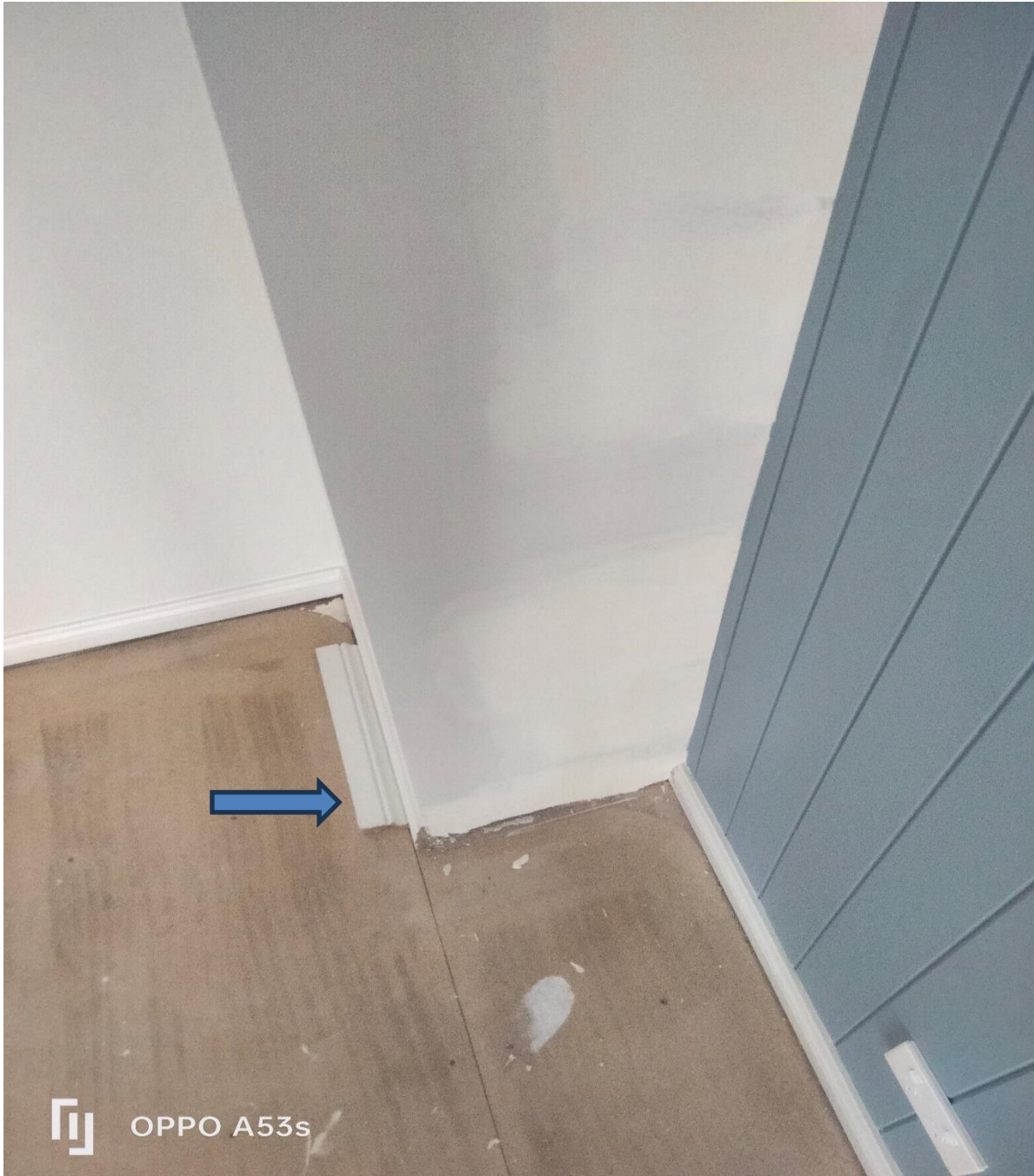
Figure 20 front main bedroom location skirtings were observed as incomplete.
