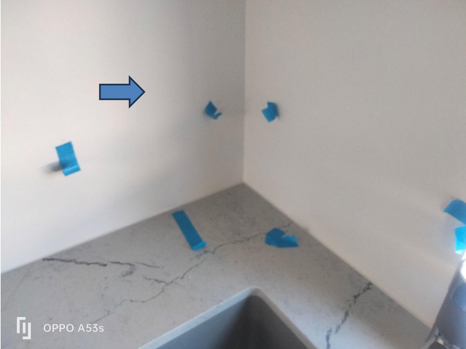
Figure 9 kitchen location wall also had painting incomplete noted. This is incomplete work.
