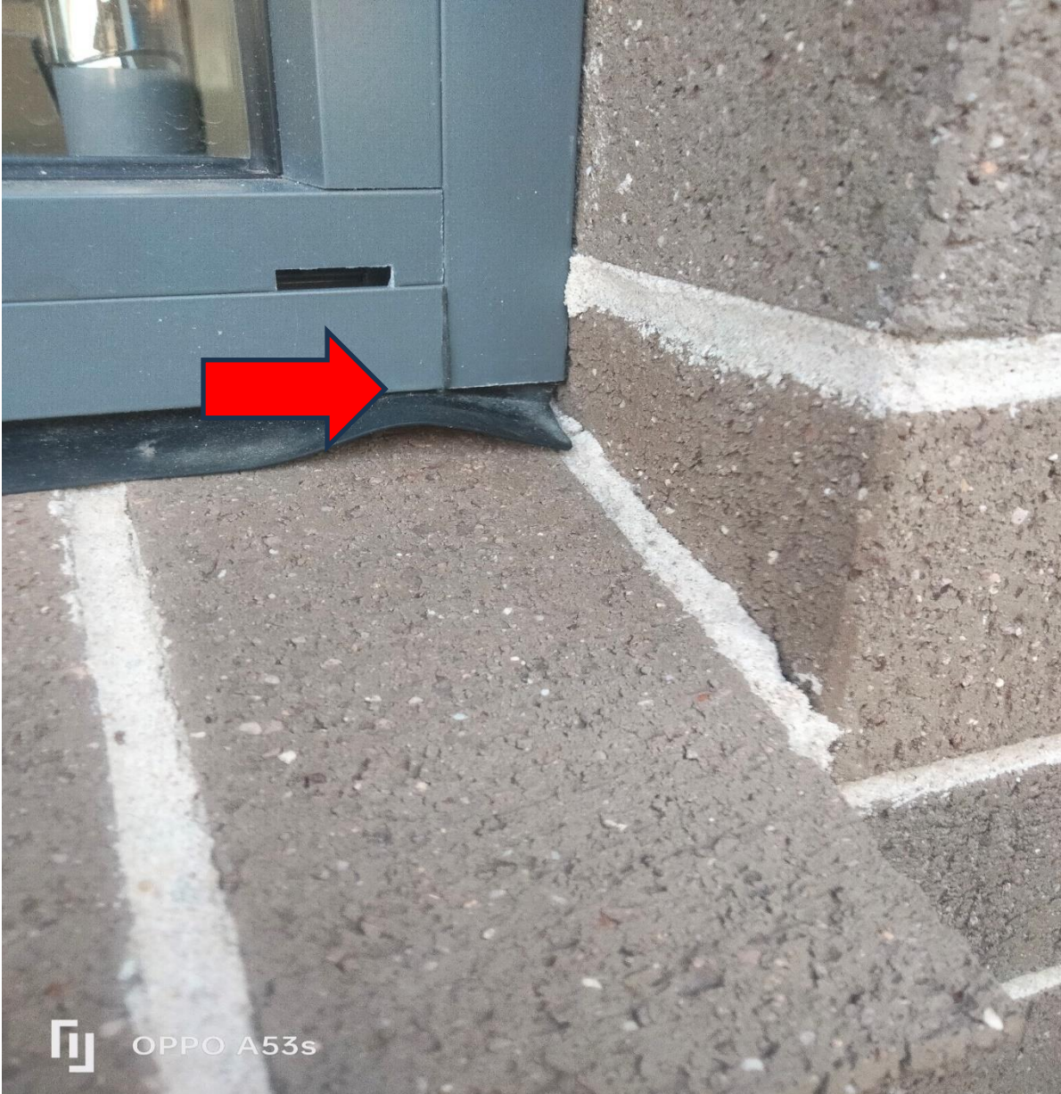
Figure 31 the window rubber seal is not installed correctly and may allow water to enter the building/.non-compliant work.
