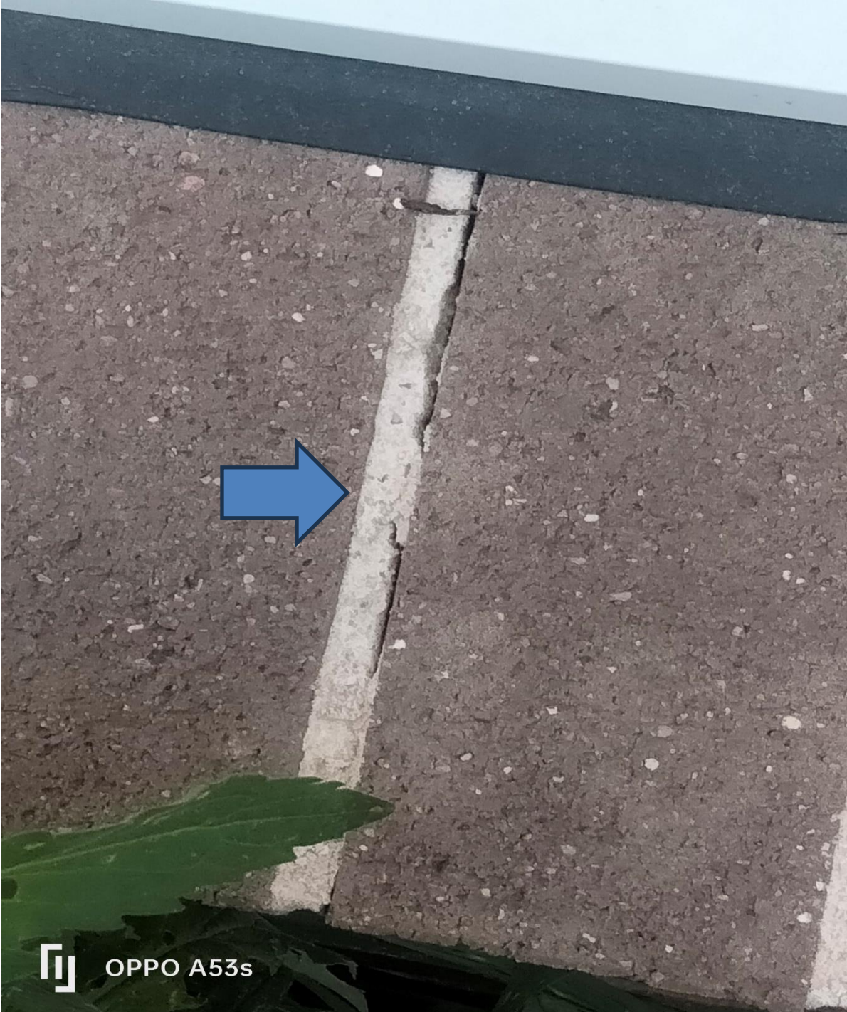
Figure 24 exterior brick work was observed as not compliant to windowsills and the exterior brick work not in accordance with NSW Fair trading tolerance Guide 2017.
