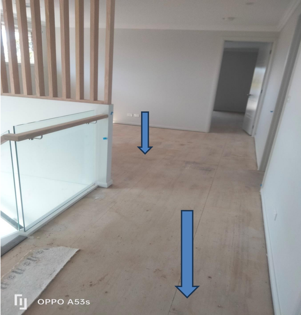
Figure 13 the first floor was observed as squeaking, this is not compliant with the NSW Fair trading tolerance Guide 2017.
