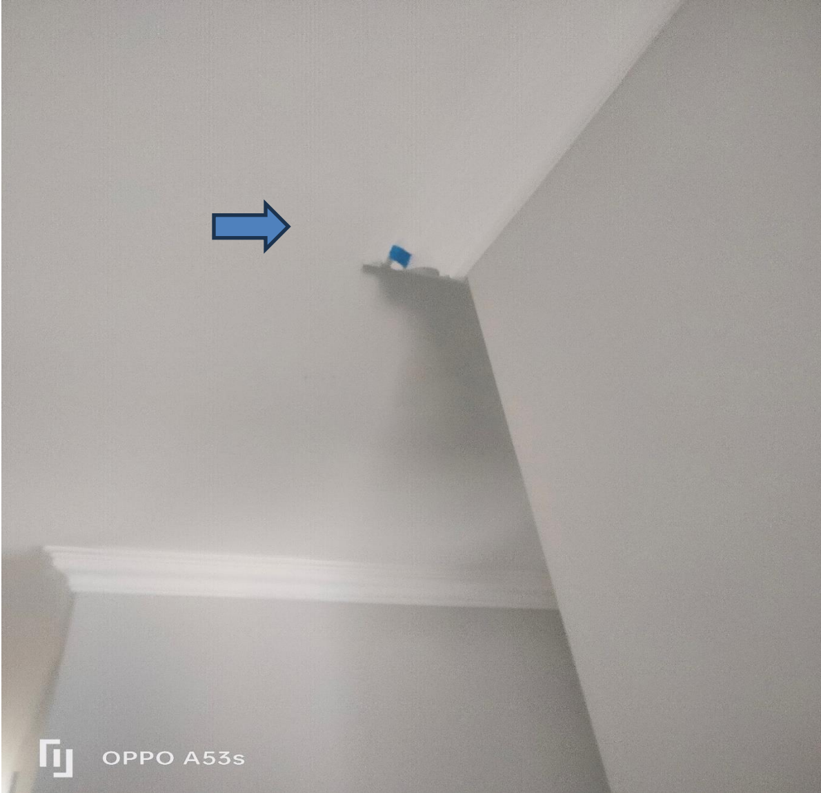
Figure 3 the interior walls and ceilings were observed as requiring final paint multiple locations. Incomplete work.
