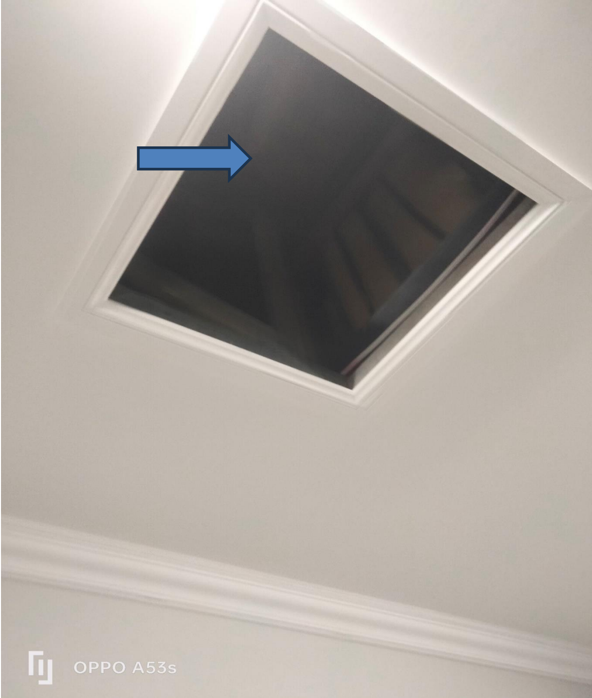
Figure 34 the manhole was observed as missing to the garage.
