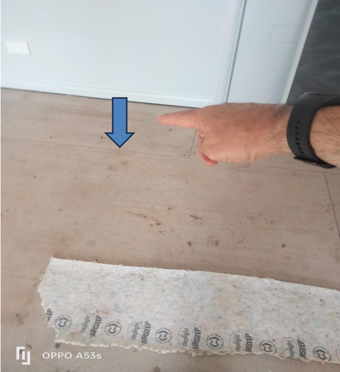
Figure 15 location top of stair landing squeak observed to the floor.
