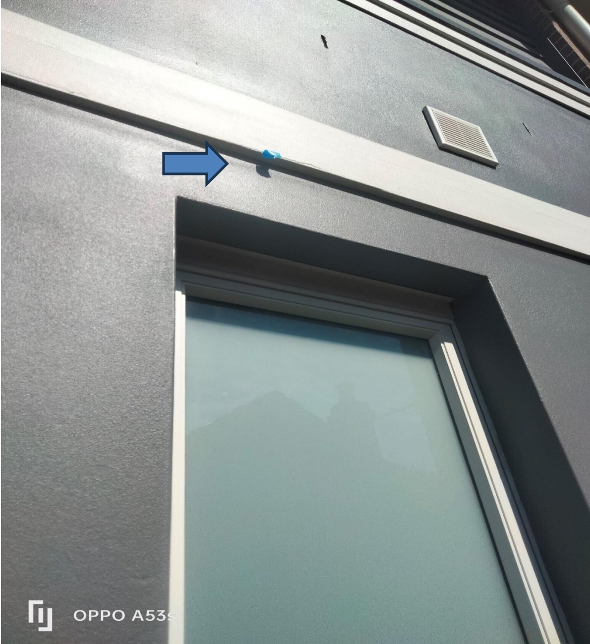
Figure 22 external render front right-hand side facing was observed as damaged requiring completion.
