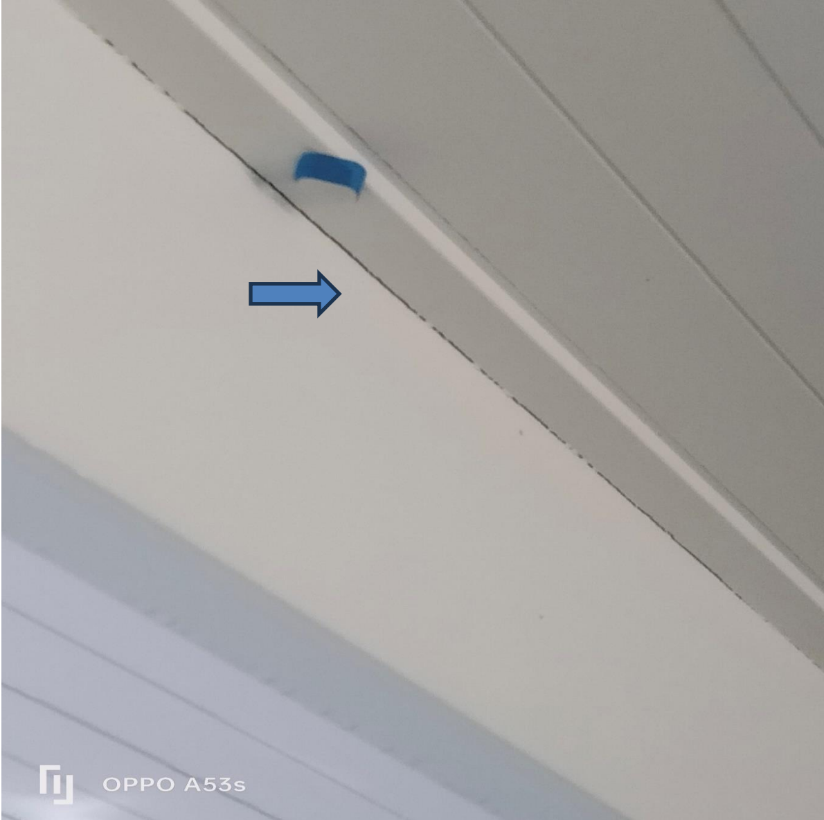
Figure 29 gap filler was observed as missing to the midpoint ceiling, incomplete work.
