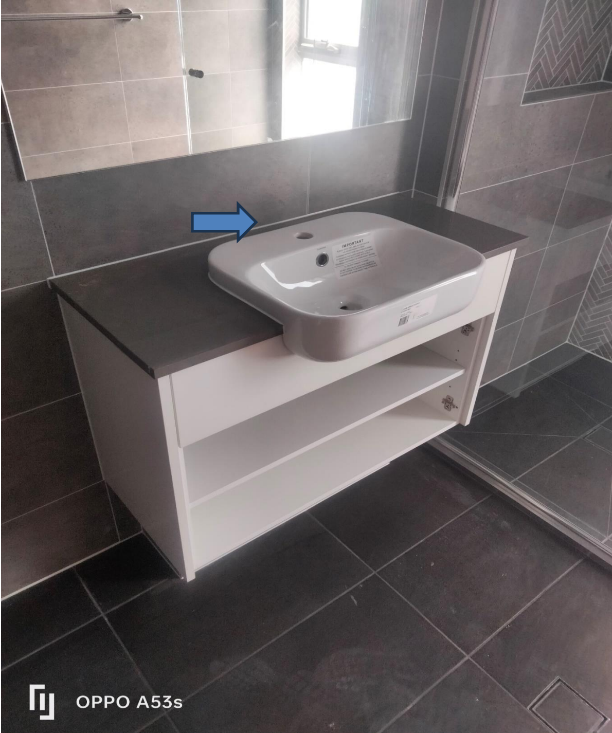
Figure 33 bathroom components were observed as missing.
