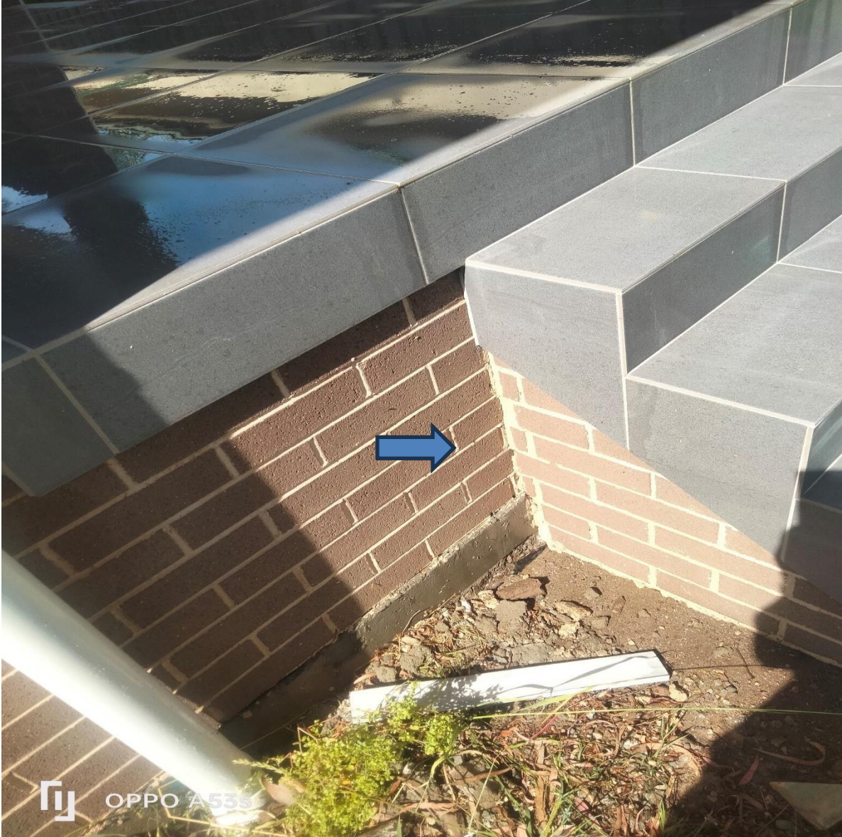
Figure 30 rear step location brick work was observed as requiring completion to the brick mortar, brick mortar was observed as incomplete.
