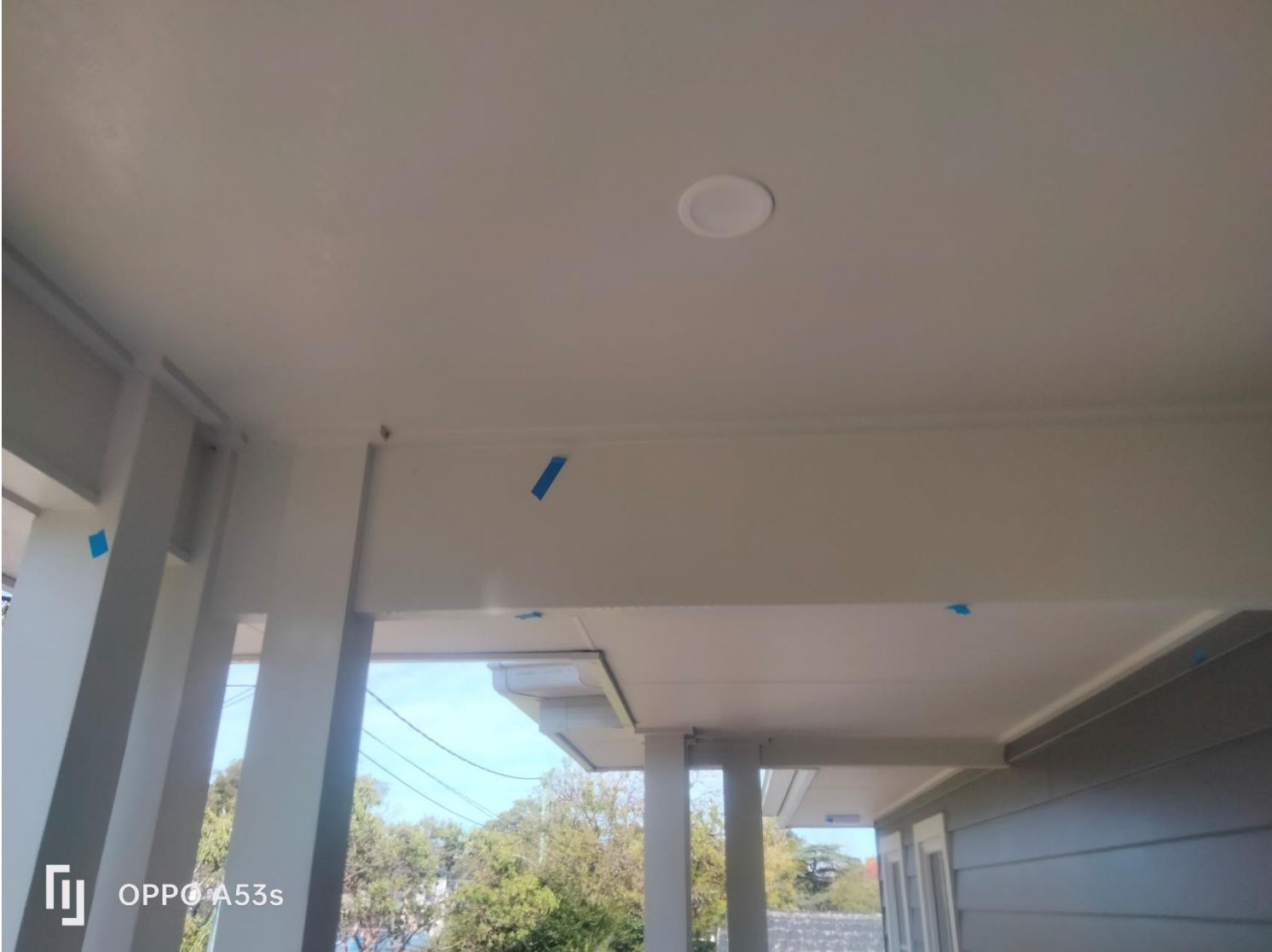
Figure 28 the ceiling to the alfresco ceiling was observed as not completed with regards to the painting, blue tape was observed indicating incomplete works.
